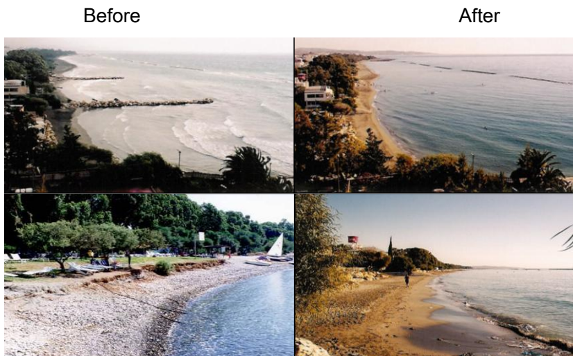
Picture 1. Demolition of groynes in Limassol- Germasogeia- Cyprus (Photos by Xenia Loizidou).
