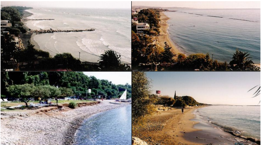
Picture 1. Demolition of groynes in Limassol – Germasogeia - Cyprus (Photos by Xenia Loizidou).
